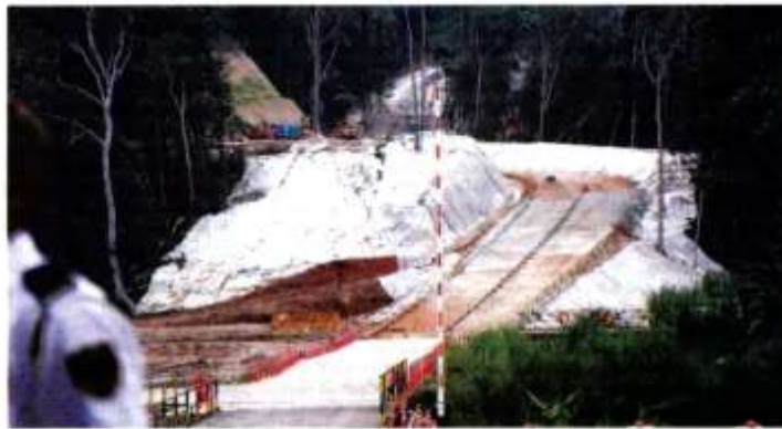
MRL has presented a definitive solution to the issue of safeguarding the Gombak Quartz Ridge by designing an alignment that traverses through an existing road for ECRL to cross the quartz ridge
